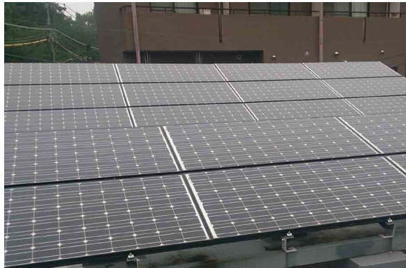
Solar powered: NSSK-backed Sakura Pharmacy Group is working to install photovoltaic power generation and energy storage facilities in its stores
